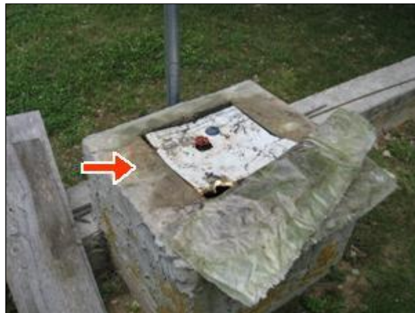
4.1 Picture 3 Well head
